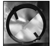
Black Tape on Damper
