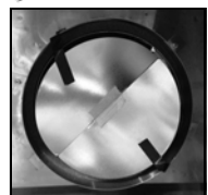
Black Tape on Damper
